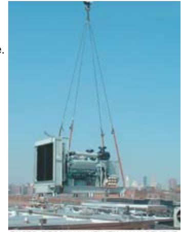
PHOTO: BROOKLYN UTILITY MANAGEMENT A 1-MW genset being hoisted high above the city skyline
